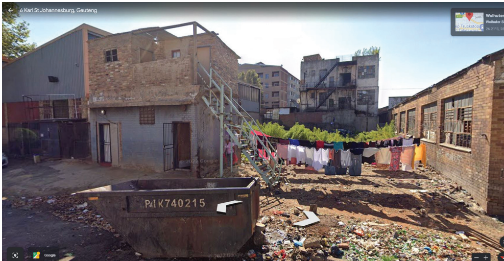
Figure 5. Here to stay: permanent, upper-storey addition in Karl Street near the Wolhuter Men's Hostel. The addition is likely to have no building approval but is not hidden, indicating a lack of municipal oversight.
